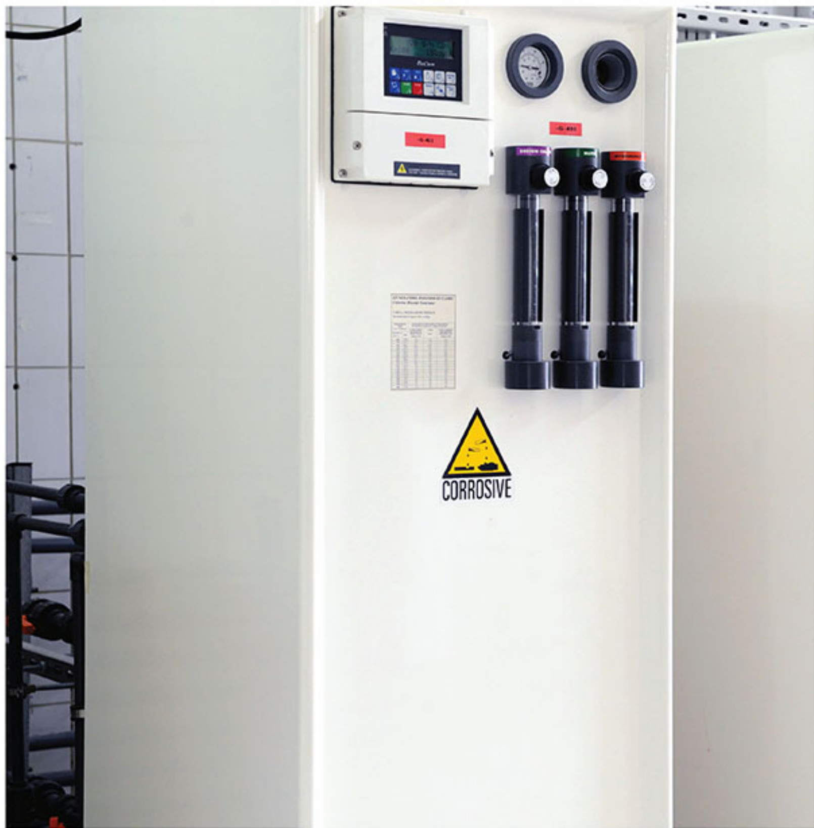
Capital Controls® G4000 Chlorine Dioxide Generator — Dubai, UAE
