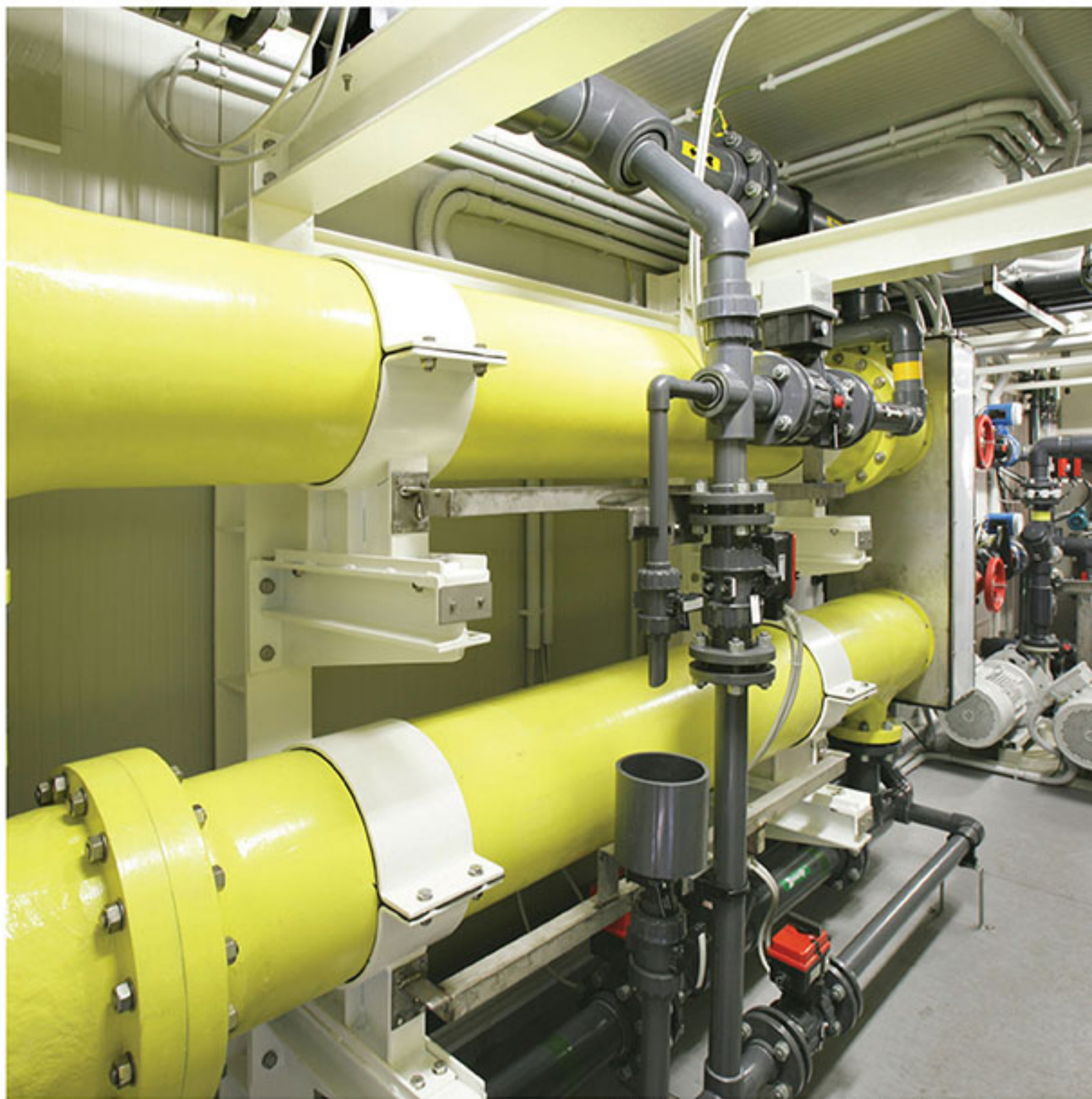
SEACLOR® Seawater Electrochlorination System installed in a power plant
